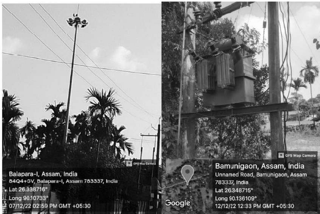
Figure 33:- Transformers and High mast light
